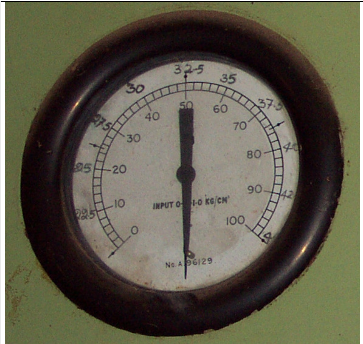
Fig. 1: MIC Storage Tank 610 Control Room Pressure Gauge
