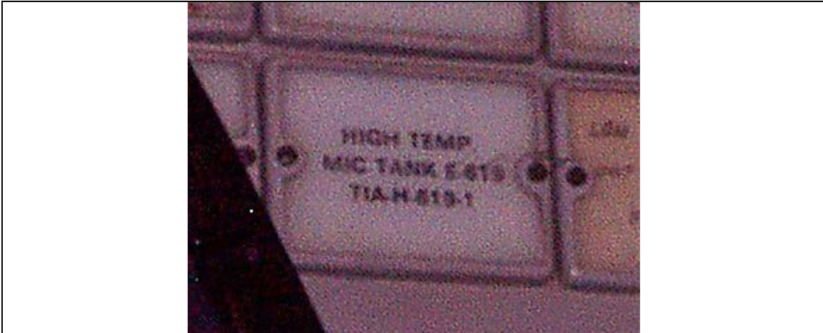
Fig. 7: MIC storage Tank 610 High Temperature Panel Alarm
