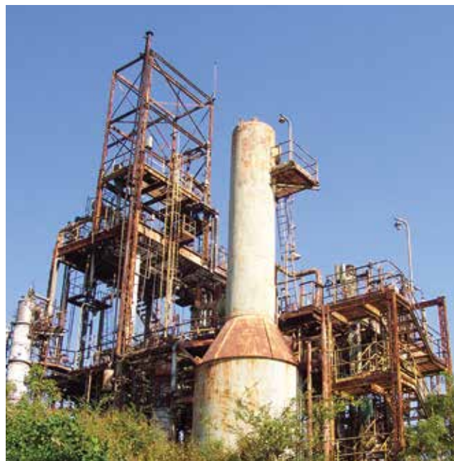
▲ Figure 6. The scrubber had been shut down for maintenance. If it were in service, it would have been overwhelmed by the volume of MIC released, as it was sized for small releases. Photo courtesy of Dennis Hendershot.
