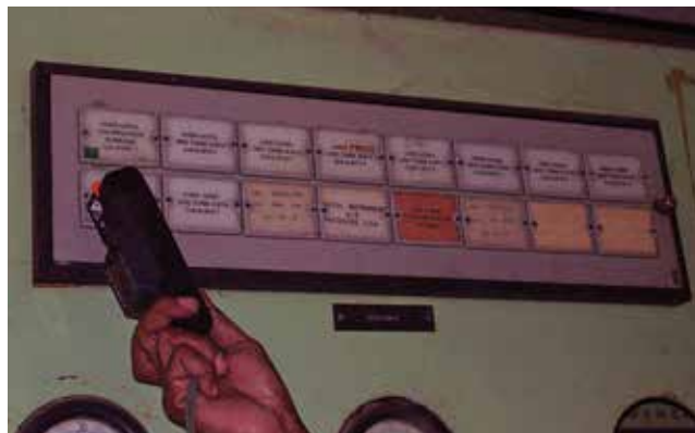
▲ Figure 5. The storage tanks were equipped with temperature and level indicators that would alert operators to abnormal conditions. Photo courtesy of Dennis Hendershot.
